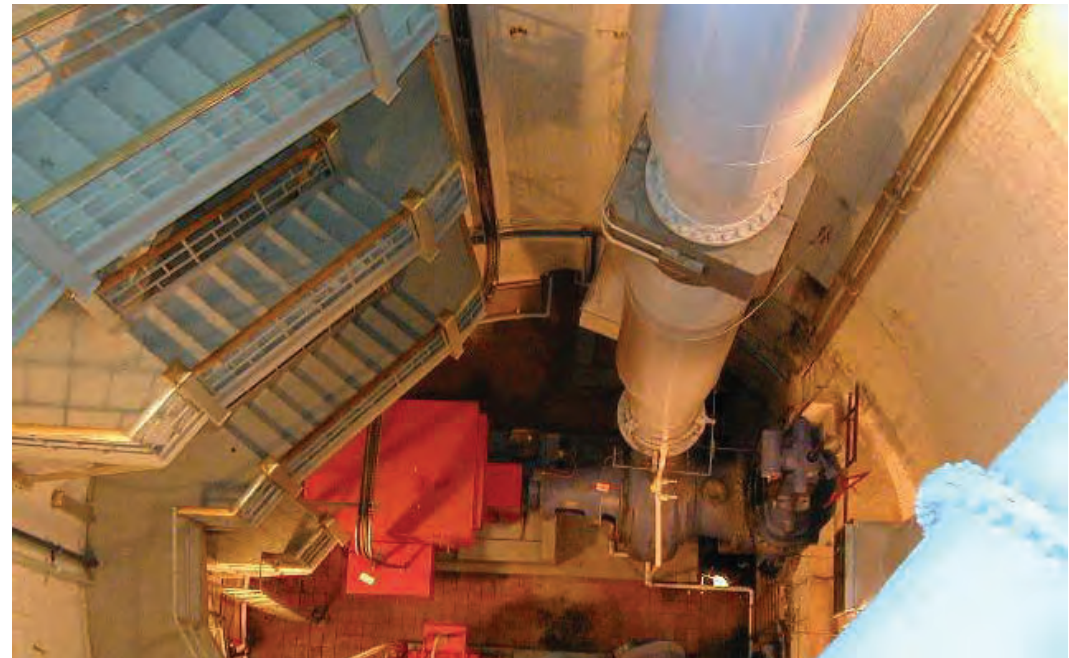
NEWPCC Raw Sewage Pumps
