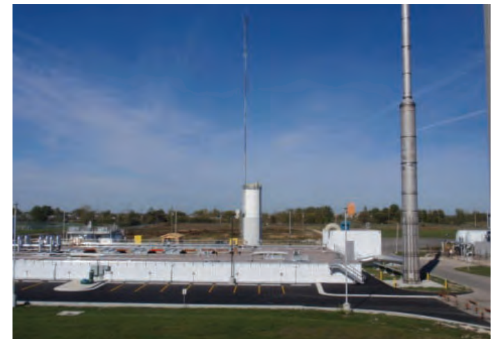
NEWPCC Centrate Nitrogen Treatment Facility
