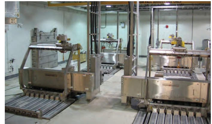
NEWPCC Ultraviolet Disinfection System
