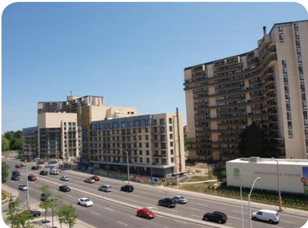
New street related construction in front of existing apartment buildings, Shepard Avenue, Toronto
