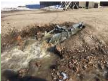
Roadside drainage ditches and damaged culverts.
