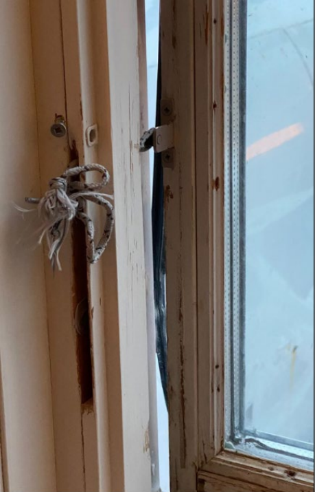
In this home, the window could no longer close. The bent window was now held with a rope, leaving a major gap that allowed in cold air, rain and snow.
