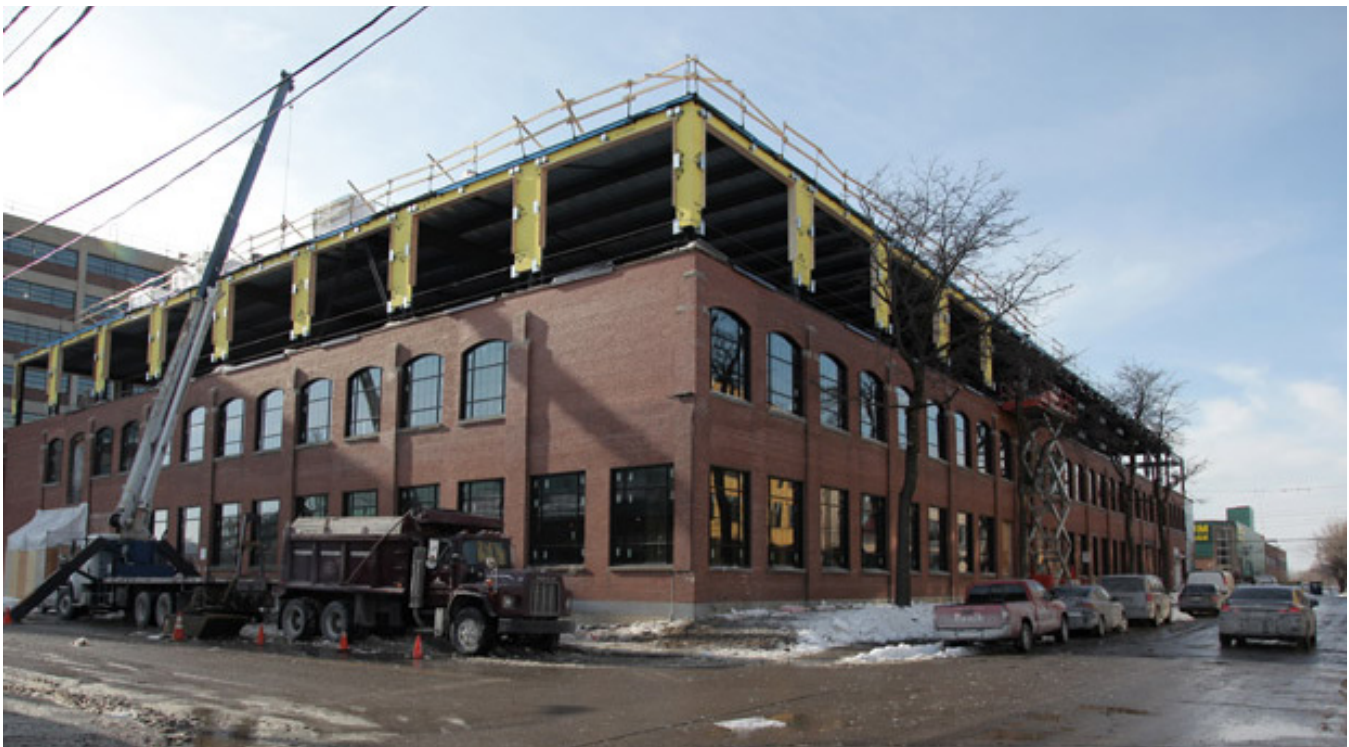
Figure 2.6. Construction of an addition underway at 7250 Rue Marconi (Case Study 2, Montreal), as the former textile factory was being transformed to an office building in 2014.
