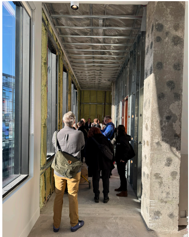
Figure 4.8. Workshop attendees at the final stop of the tour, the penthouse of 1660 Hollis Street (Case Study 1) where construction is still in progress.
